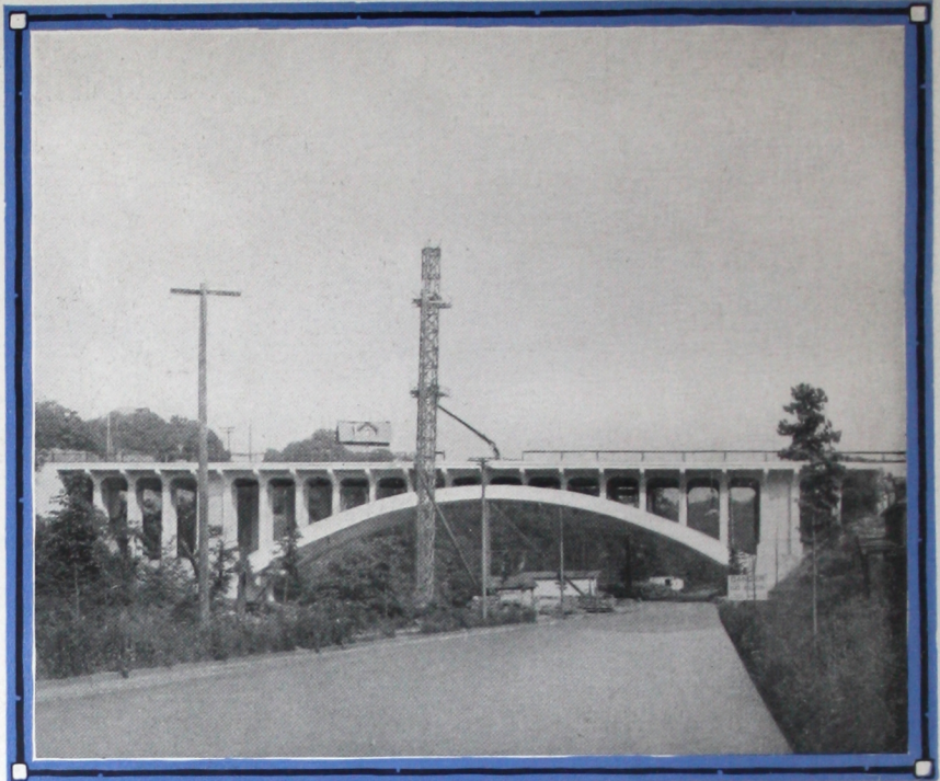
Murray Avenue Bridge, Pittsburgh, Pa. An example of open spandrel walls ALPHA CEMENT used
