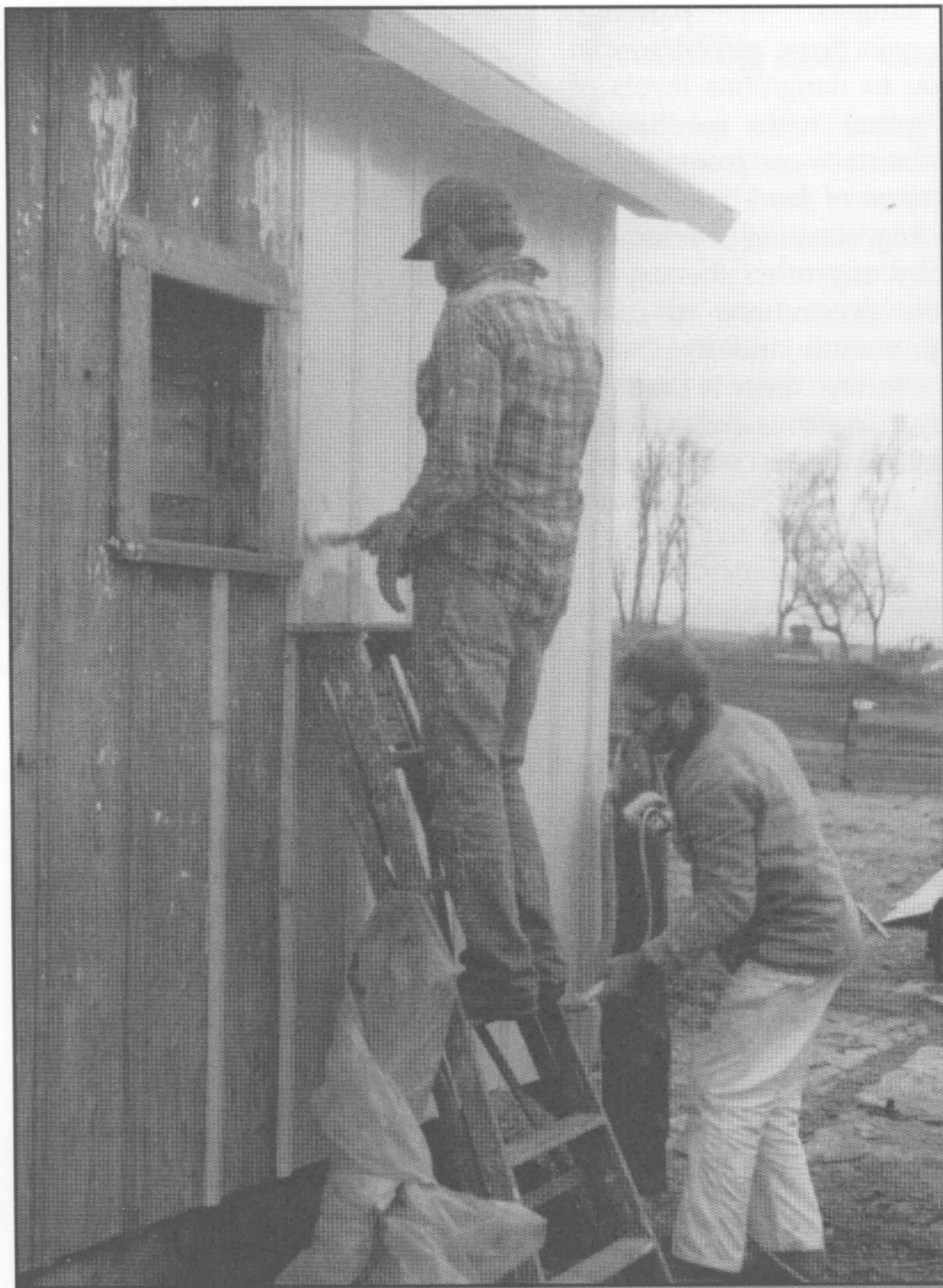
Primer is applied to barn with power sprayer, then brushed into the wood to ensure thorough penetration.
