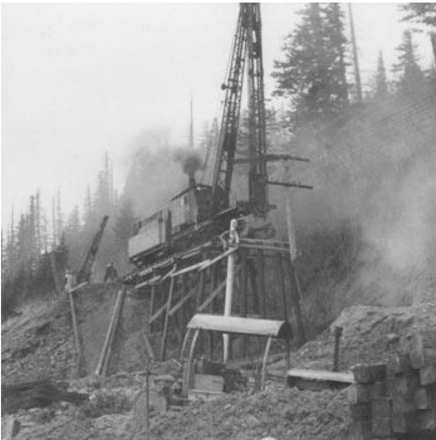
Figure 10. A pile driver work on a trestle during the construction of the SP&S. Source: SP&S 700 Pacific Railroad Preservation Association.
