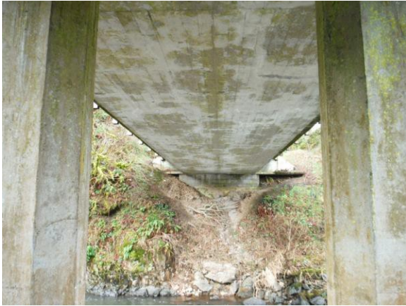
spalling visible on underside Underside of box girders, concrete pillars 2015
