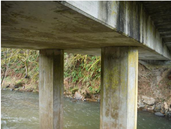
Cast-in-place reinforced concrete pillars, underside of box girders Underside of Bridge 65, looing west/southwest 2015
