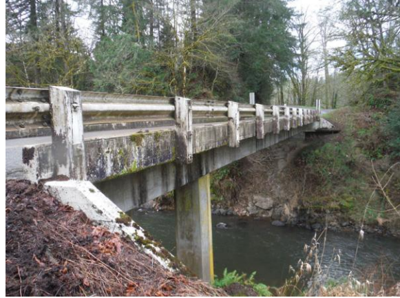
Metal and wooden guardrail, cast-in-place concrete pillar north side of Bridge 65, looking west 2015
