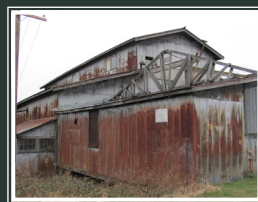
REID BOILER WORKS Built in 1912, the building houses the Reid Boiler Works. Founded in 1899, the company supplied
