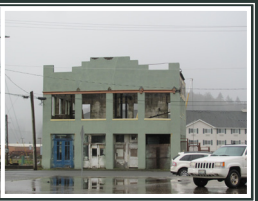
BREAKWATER SEAFOOD BUILDING Built in ca. 1905, the former Breakwater Seafood Market is one of Aberdeen's oldest buildings. Originally a logging company office, it later became a seafood market. Damaged by fire in 2007, it is under renovation.
