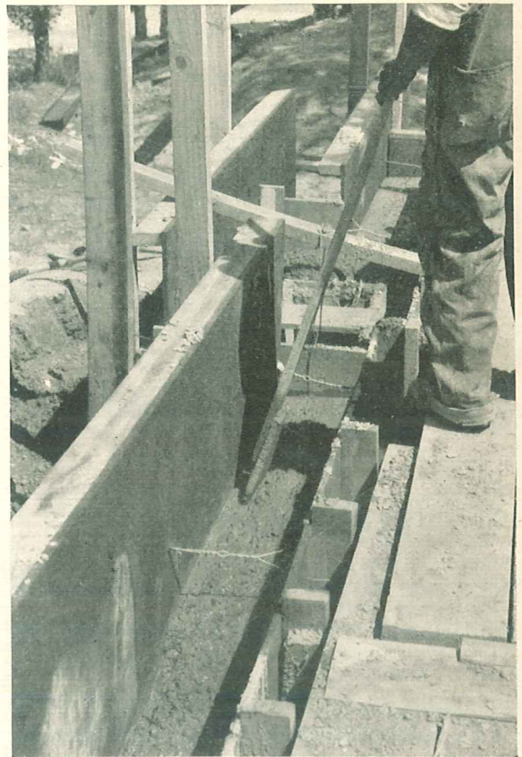
Thorough spading of concrete along form faces helps assure smooth, watertight concrete walls.
