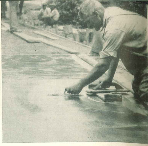
Right —Concrete floors should never be finished until the concrete has hardened enough to become quite stiff. The wood float is used for final finishing if a gritty, nonslip surface is desired. For smooth, dense surfaces, use the steel trowel for finishing.
