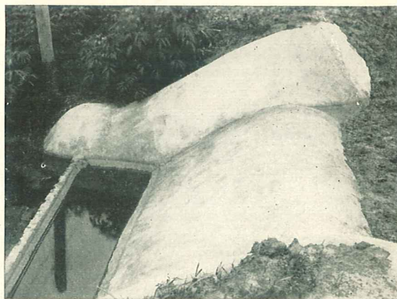
This low-cost concrete flume is constructed by placing a 5-in. thickness of concrete on a carefully formed slope.
