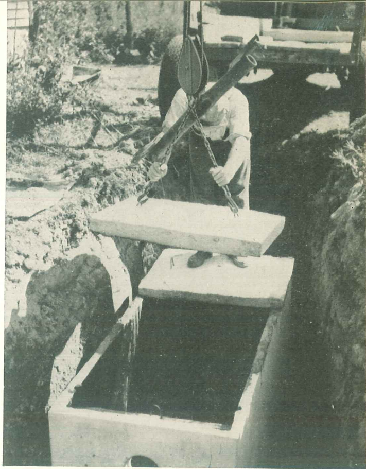
Precast concrete septic tanks are available in some localities. Here is one being delivered and installed. Family-size precast tanks should have a minimum working capacity of 500 gal. and should provide for a sewage depth of at least 4 ft.
