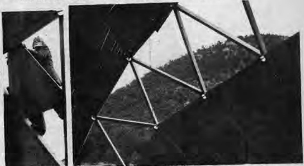
Skinning the dome was a special problem, since the triangles were all too large to cover with single sheets of plywood. We used small 3/4" and 5/8" CD plywood triangles inverted inside each triangle of struts, and then filled in the 3 corner triangles that this created with 1 X 4"s. The 1 X 4"s were cut on jigs and hauled up in numbered sets to be nailed in place.
