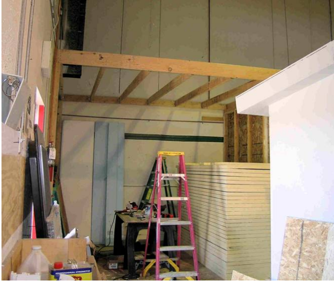
The chamber was framed into the corner of a warehouse. The existing walls were first covered in two inches of polyisocyanurate (R-13).
