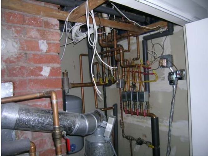
Multi-zone heating system
