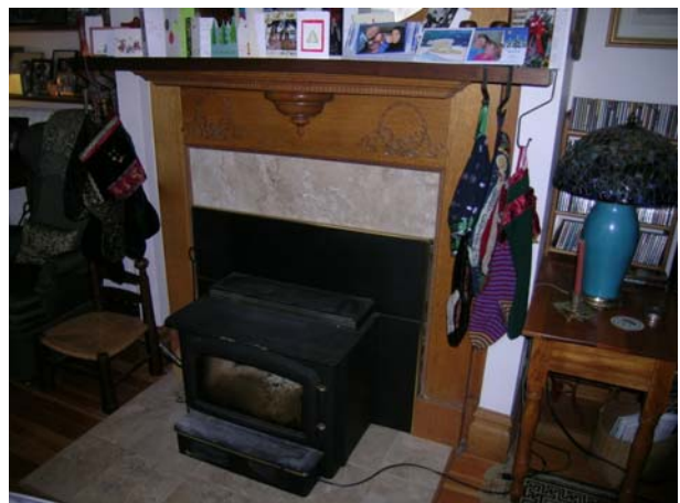
Wood stove vents into existing chimney
