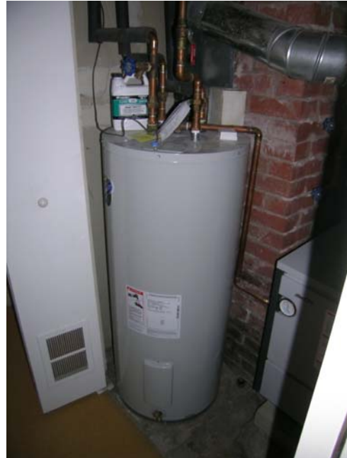
Domestic hot water tank
