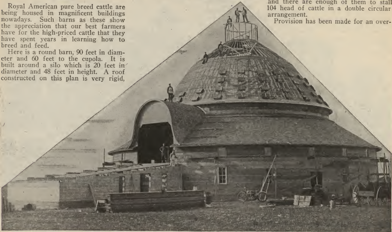
Ninety foot round barn, No. A254L, in process of construction in Iowa. Roof is sheathed with \frac{7}{8} by 2-inch strips. Horse stable is concrete block section under bridge to hay mow floor.
