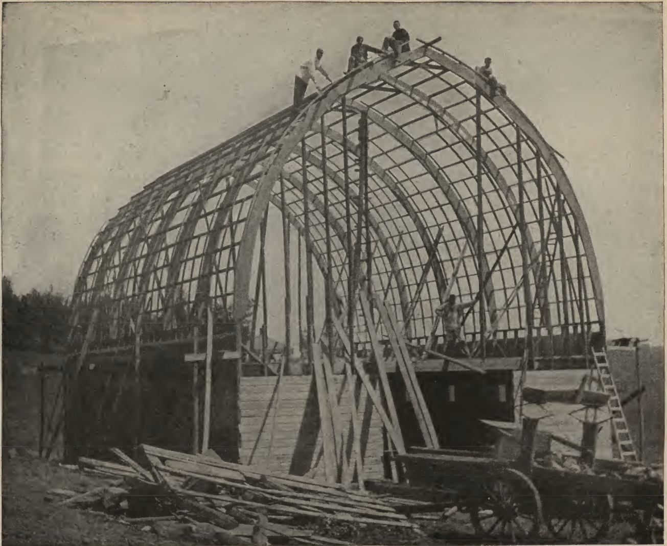
Photograph taken during construction in Washington of Gothic roof barn, Design A280L. Notice how main rafters are constructed; the curve is sawed out of 12-inch boards and these segments are nailed four together, breaking joints.
