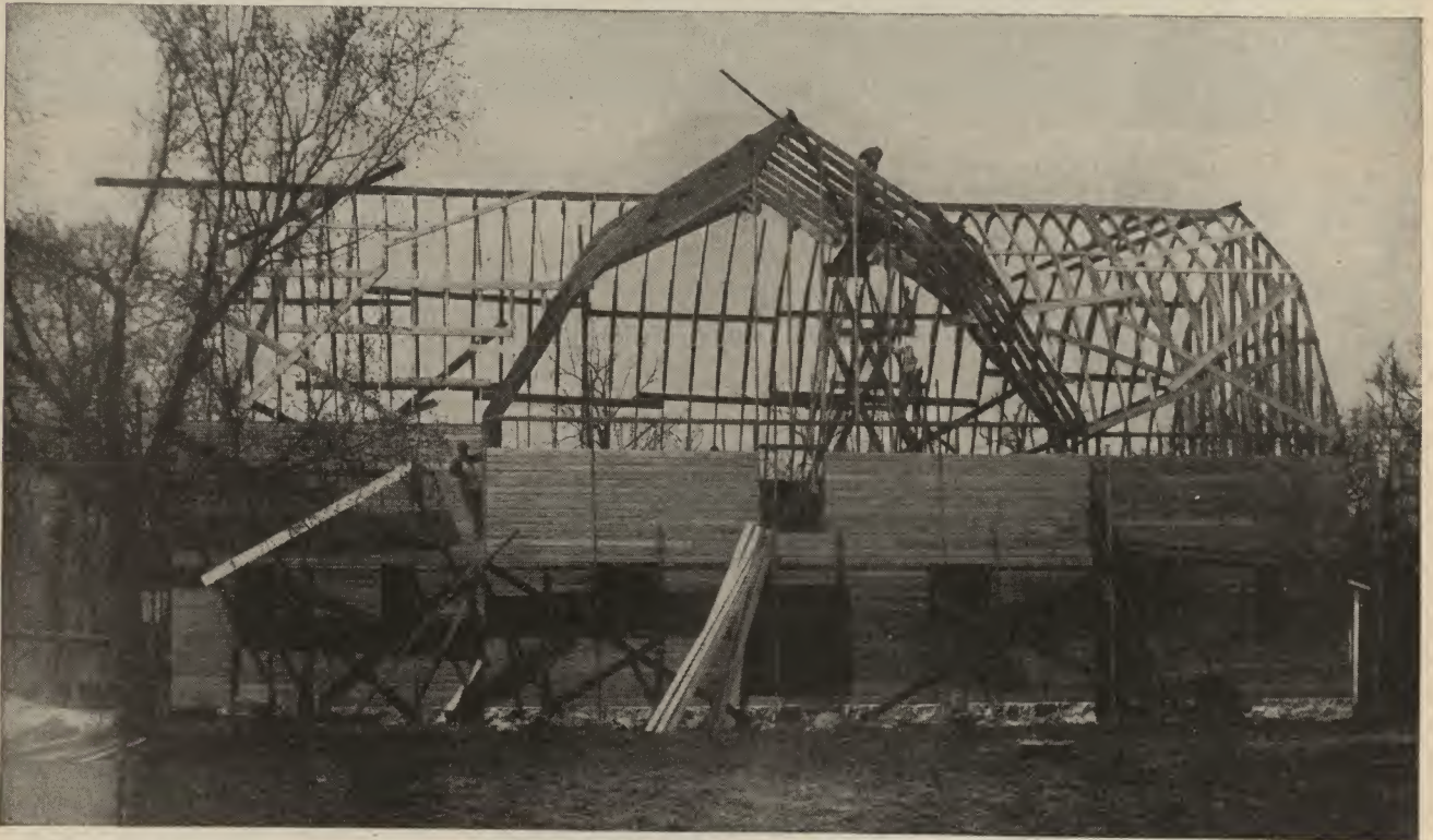
View of North Dakota General Farm Barn, design No. A261L, taken during construction. Note how rafters are framed for 36 foot full-height gambrel dormer. This gives an immense space for hay storage, besides strengthening the roof.
