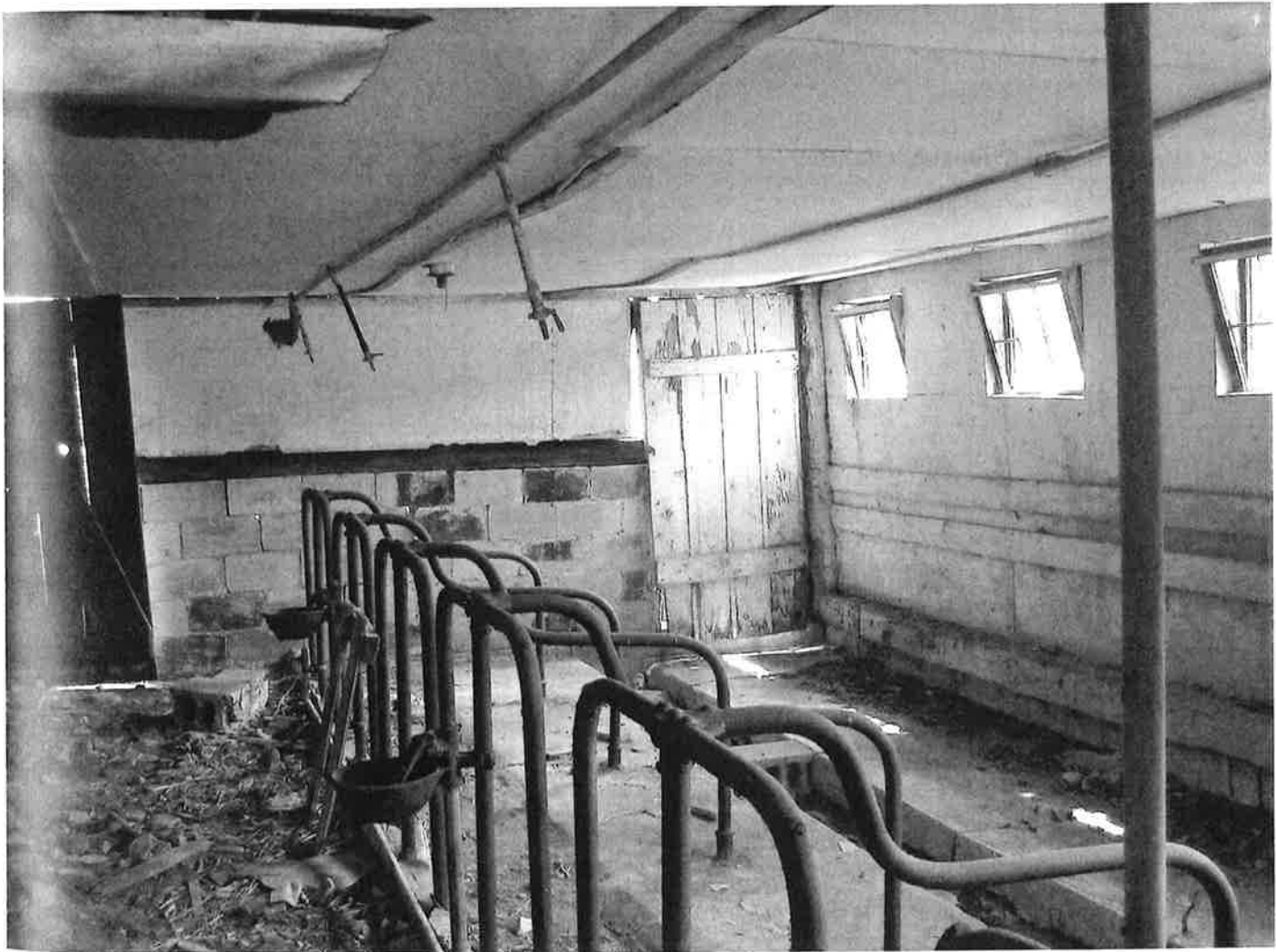
Figure 8. Interior barn renovation, Tioga County, Pennsylvania. This late nineteenth-century barn stable was renovated around 1930. Concrete floors and metal stanchions with water cups were installed, and tilting metal windows were inserted into the stable wall. Photograph by the author, 2008.
