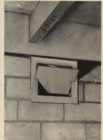
This shows the interior view of the Fresh Air Intake installed in a block wall.
