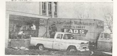
Heavy Warehouse Deck Now Tearing Highway's Offices Building
