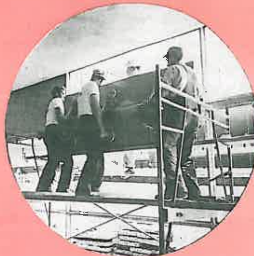
Assembled panel is installed with suction device at job site. Prefabricated panels helped cut construction time and costs.
