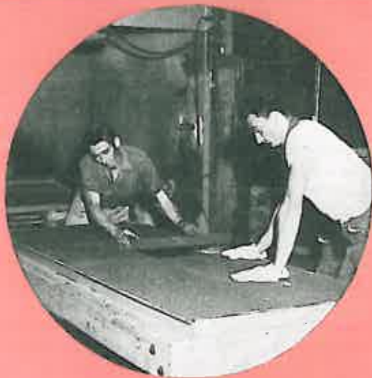
Enamelled steel wall panels were prefabricated for job. Here, Foamglas insulation is installed in panel at Beaver Falls, Pa.
