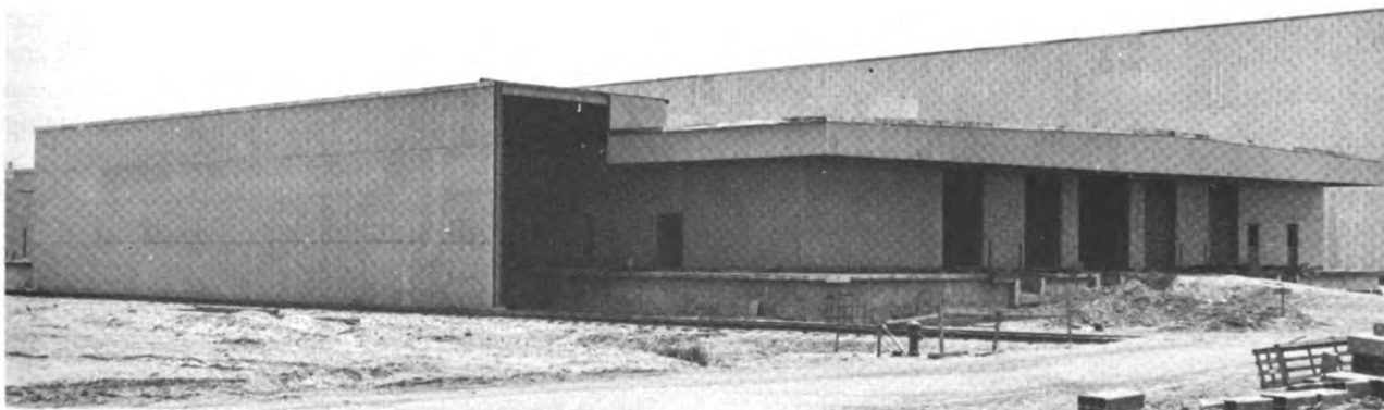
Fig. 4.17—Cornice flashing of stainless steel is used with porcelain enamel on the general stores building.
