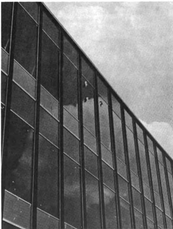
Fig. 1.6—Glass and porcelain enamel panels in place in "curtain wall" of the administration building in the engineering group of the General Motors Technical Center, near Detroit, Michigan.
