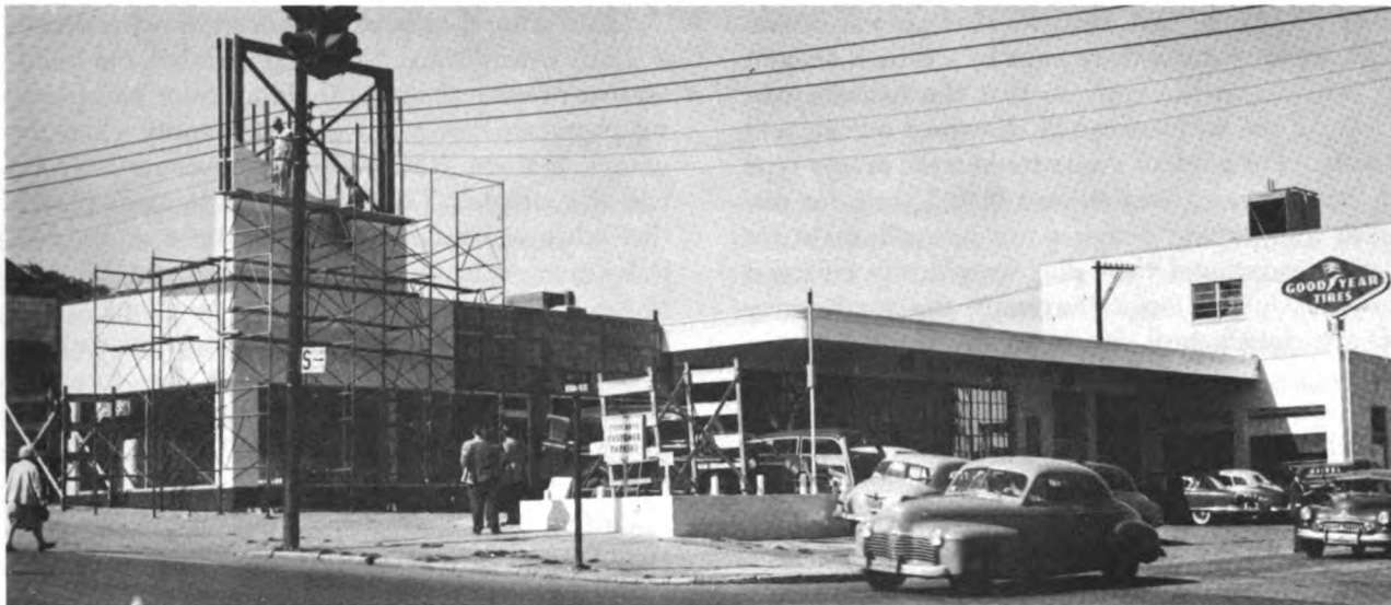
Fig. 4.7—Cook Bros. Goodyear Dealer and service station in Akron, Ohio in process of construction with porcelain enamel finish.
