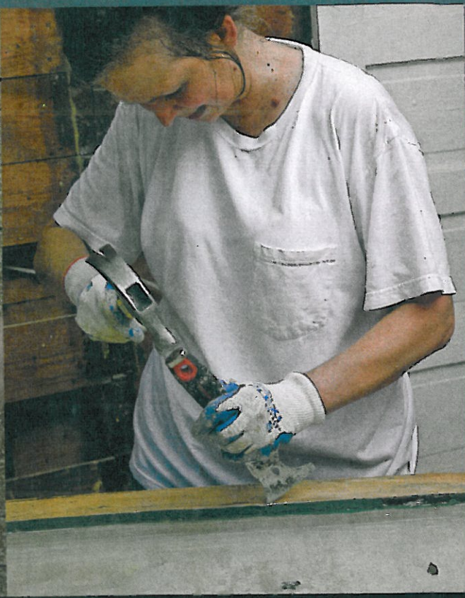
Pam carefully removes glazing compound (which had been painted green along with the window frame) from the sash.
