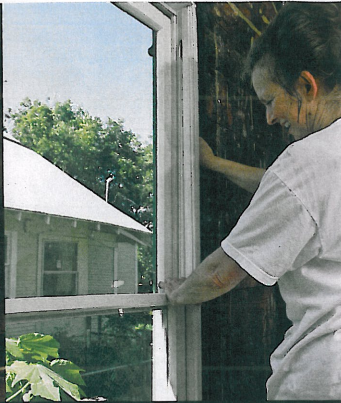
Once both sashes are in place, Pam checks the rope again and adjusts as necessary before replacing the interior stops and trim.
