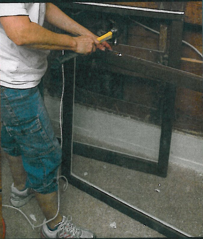
Pam nestles sash rope into an existing hole, then hammers it in place. The length of the rope fits into a routed channel along the sash.
