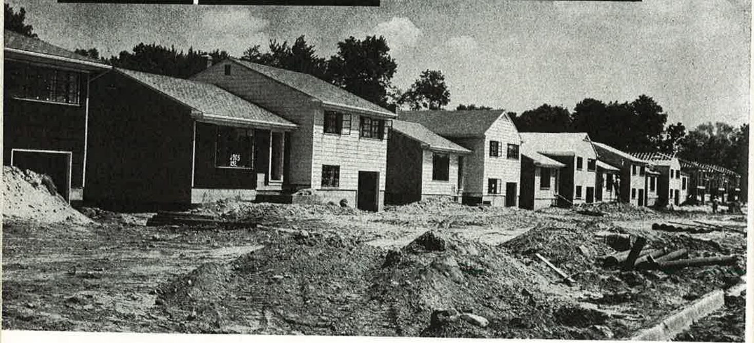
Split-level construction scene typical of today's market in the New York City suburbs. It is in Glen Crest Manor, Glen Rock, N. J.
