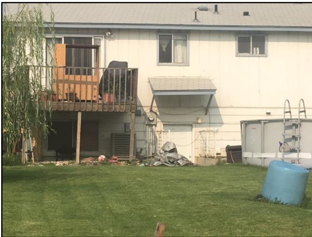
Figure 32. Close up of rear entry and deck at 727 S Douglas Avenue.
