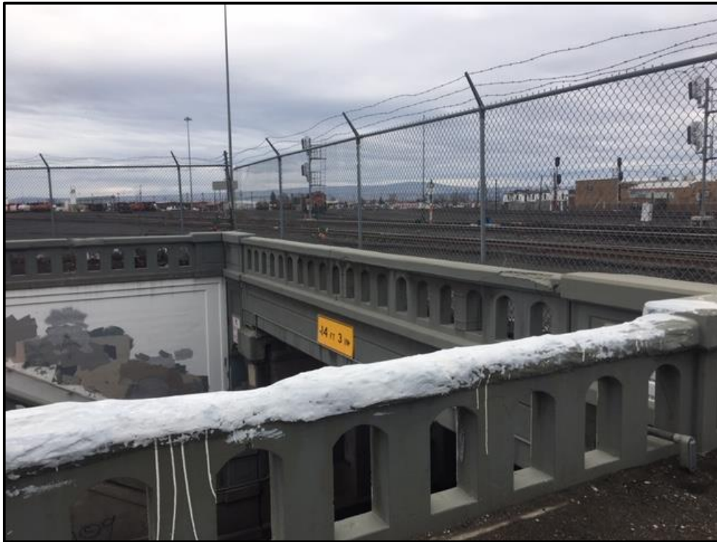
Figure 90. Photograph of the arched railings on the eastern side of the Lewis Street Underpass, looking west/northwest.
