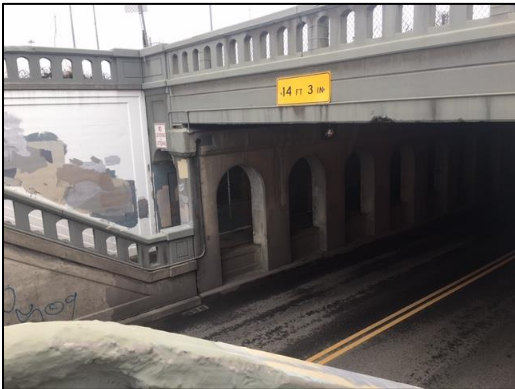
Figure 91. Photograph of the arches on stairway railings and on the concrete divider between the pedestrian walkway and the roadway, looking south/southeast from the east side approach.
