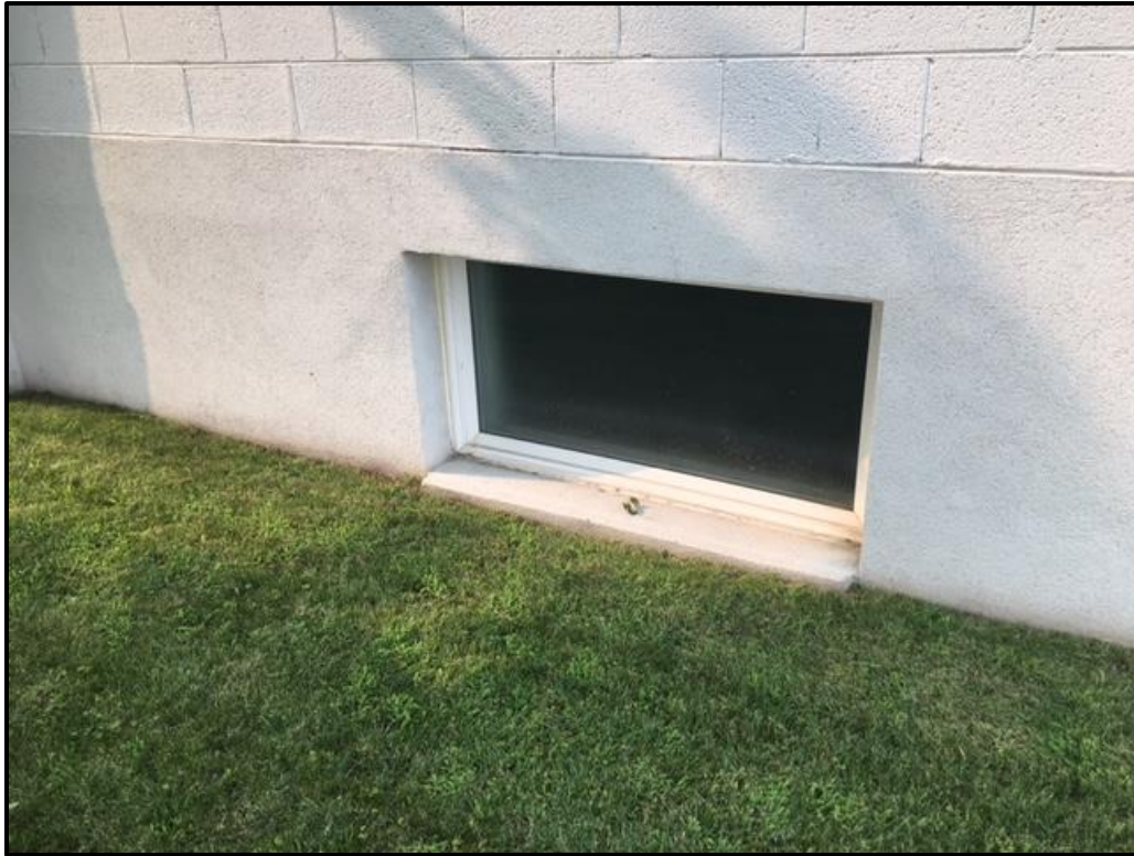
Figure 54. Detail of the basement windows along the southern elevation of the church.
