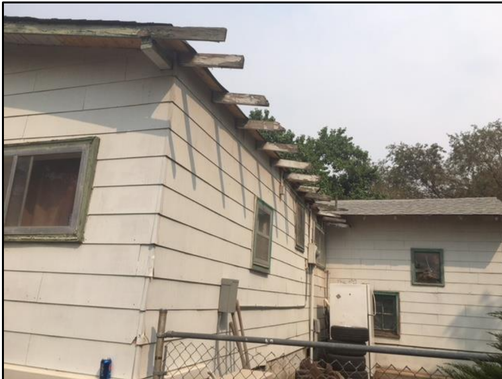
Figure 18. Exposed wooden rafters, wooden soffits and clapboard siding on southeastern corner of residence, looking north.
