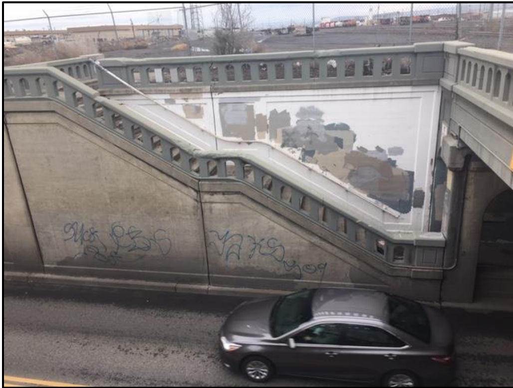
Figure 95. Patched graffiti on the east side approach to the underpass, looking south.
