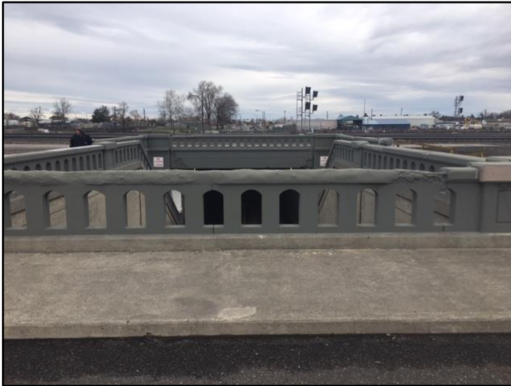
Figure 94. Photograph of patched railing on the western approach to the underpass, looking east.
