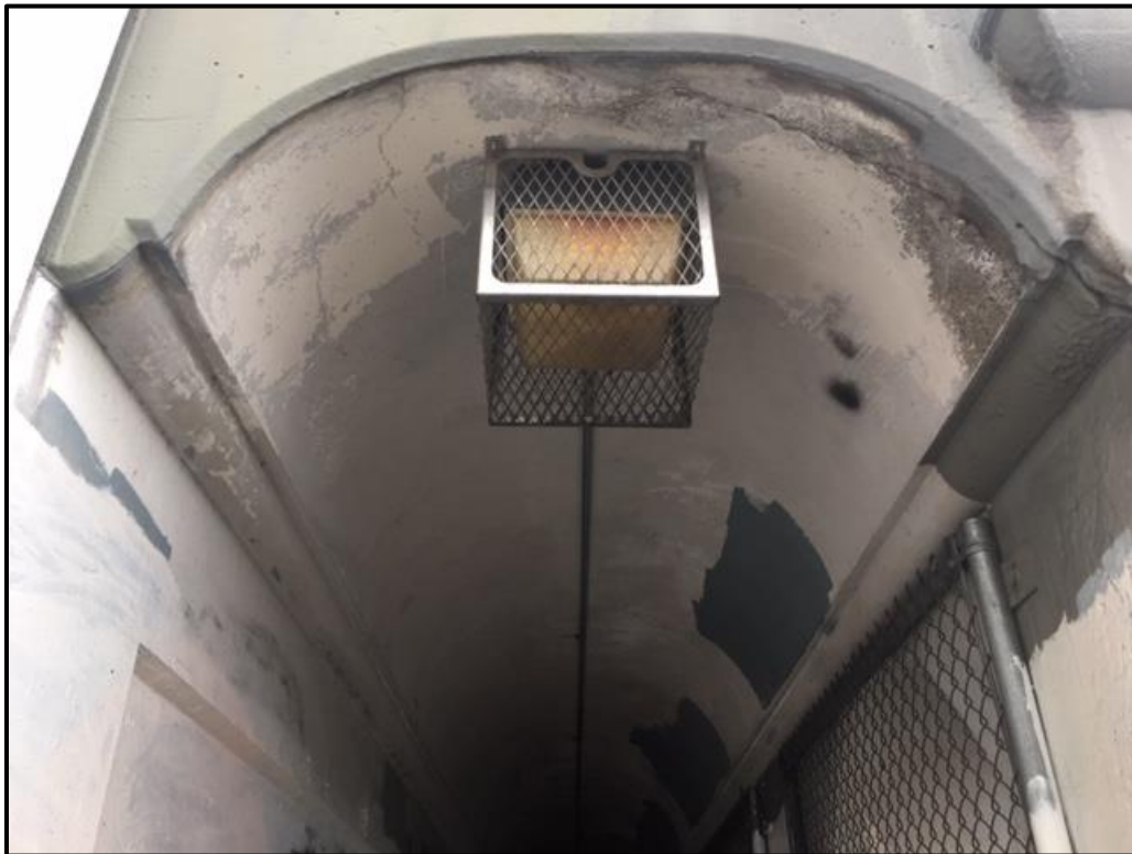
Figure 96. Electrical lighting and patched graffiti on the ceiling on the pedestrian walkway.
