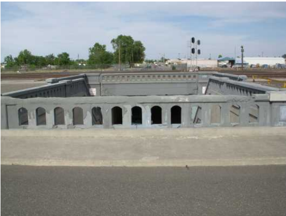
the pedestrian access of the Lewis Street Railroad Underpass at Tacoma Ave., facing east.
