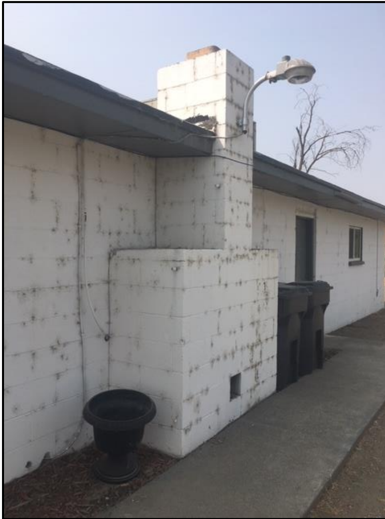
Figure 44. Detail of the chimney on the northern elevation of the Greater Faith Church building.
