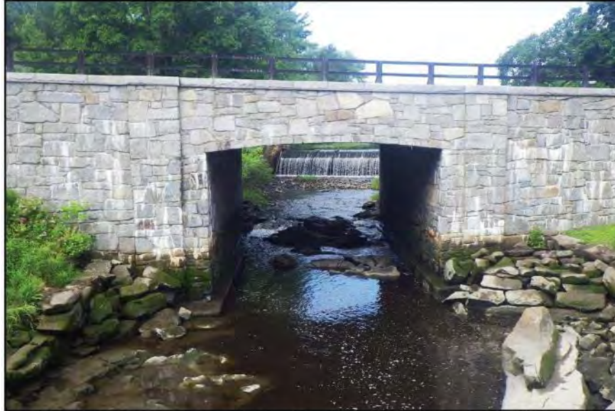
FIGURE I-51: Oyster River Bridge Replacement, in Durham, NH. Replacement Design Exhibits Retention Of Scale (Courtesy of New Hampshire DOT 2019)
