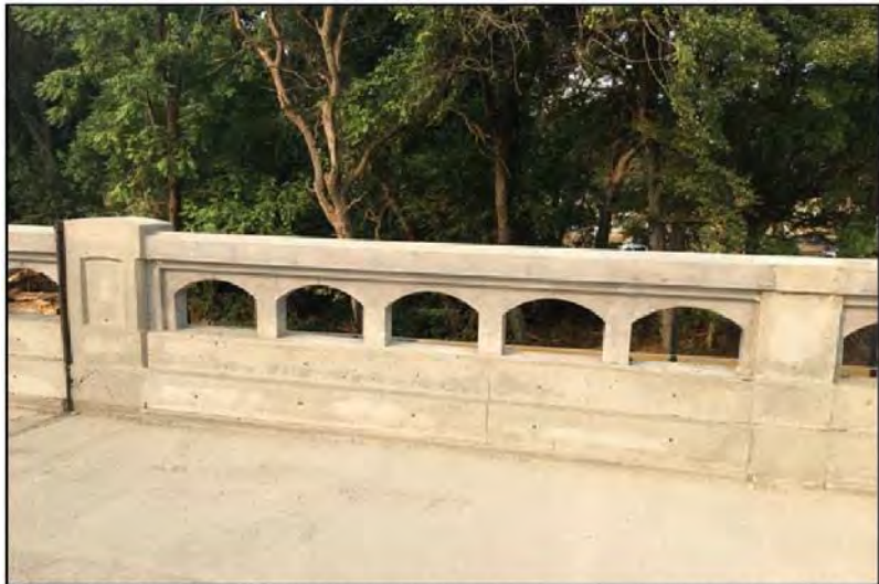
FIGURE I-46: Chenoweth Creek Bridge Replacement, Wasco Co., OR (Courtesy of Oregon DOT 2019b)
