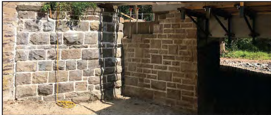
FIGURE I-38: View of Abutment and Wing Wall Construction with Cut Ashlar Stone Facing, 2017 (Courtesy of UE 2019)
