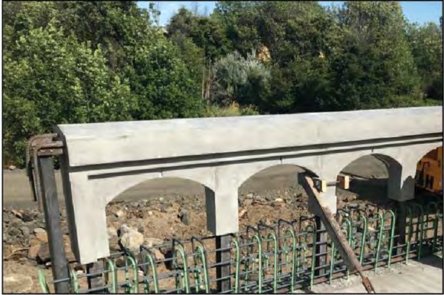
FIGURE I-7: During Construction of the Chenoweth Creek Bridge Stealth Railing, Summer 2018 (Courtesy of Oregon DOT 2019b)
