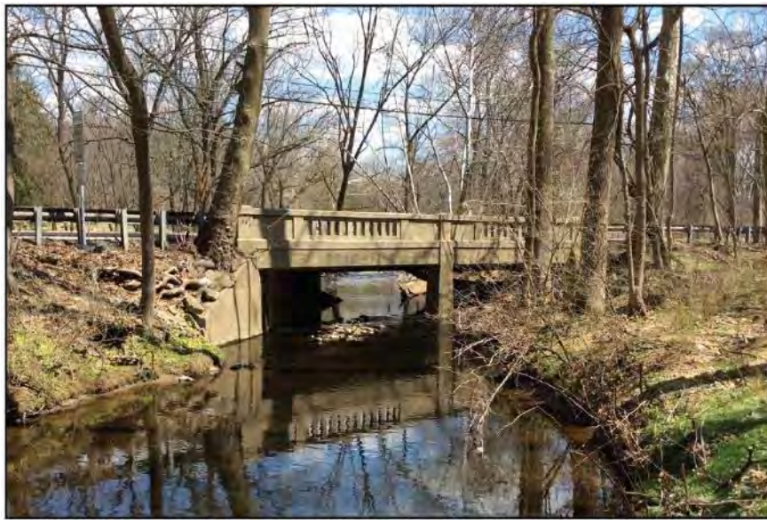
FIGURE I-10: 1927 Concrete T-Beam Bridge, Montgomery County, Pennsylvania (Replaced In 2019) (Courtesy of PWKP 2018f)
