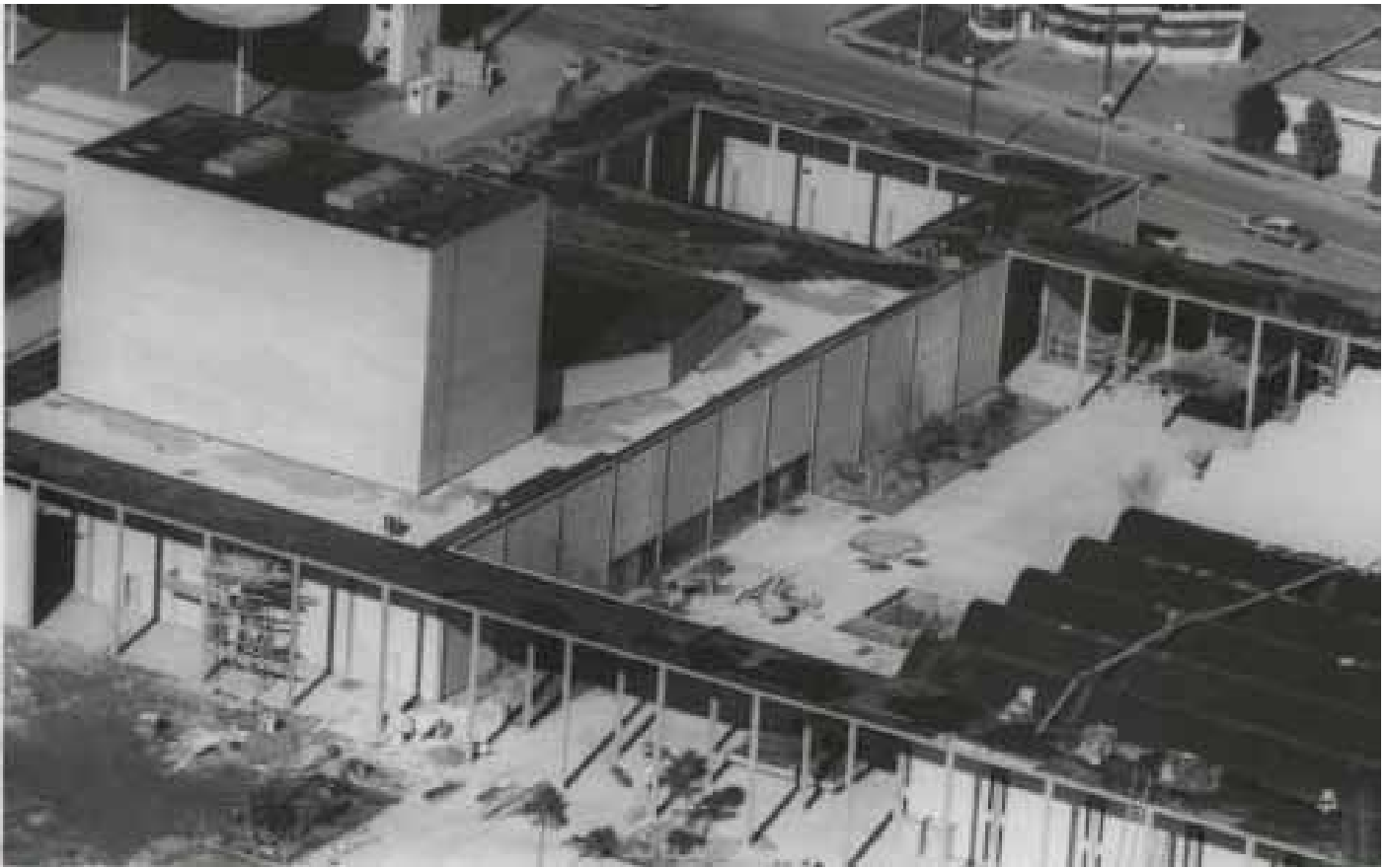
Aerial view of Playhouse and Exhibition Hall in the last stages of construction. Source: Seattle Public Library.
