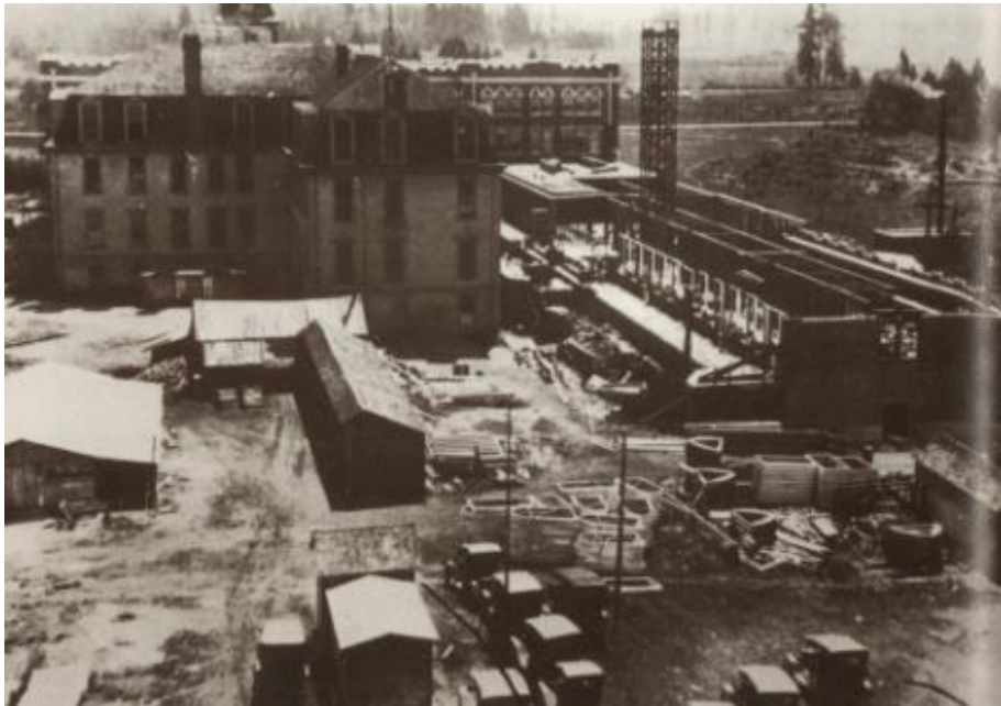
Figure 15. Saint Martin's College – Construction of west wing, c. 1920 (Image courtesy of Saint Martin's Abbey Archives, photo by Albert Fisher)
