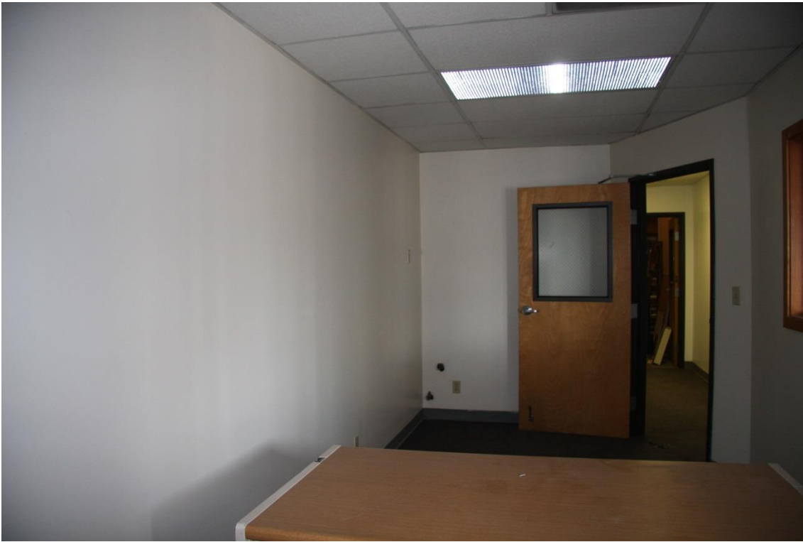
Photo #14 of 15 (WA_PierceCounty_RentonWoolworthBld_0014) Second floor interior, office, west (left) and north (right) walls, camera facing north
