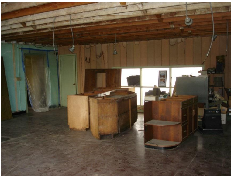
Name of Property: Luepke Florist City or Vicinity: Vancouver County: Clark State: Washington Photographer: Holly Chamberlain Date Photographed: 11 July 2015 Description of Photograph(s) and number: interior of upper floor office space in 1946 addition looking south
