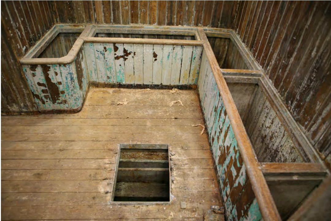
9 of 20. Western Flyer. Deckhouse, detail view of galley's built-in bench seating (seats temporarily removed).
